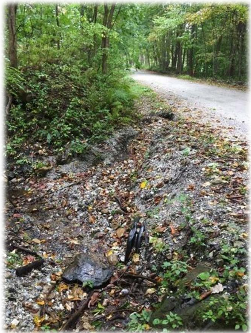
Figure 10: West Hill Road 5. The turnout at the bottom of the road is eroding directly into the tributary.
