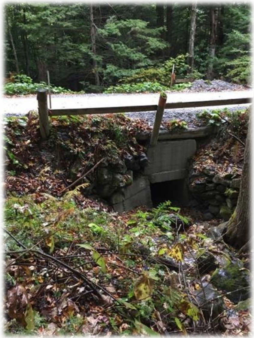
Figure 12: West Hill Road 1. Misaligned and undersized culvert at bottom of road segment.
