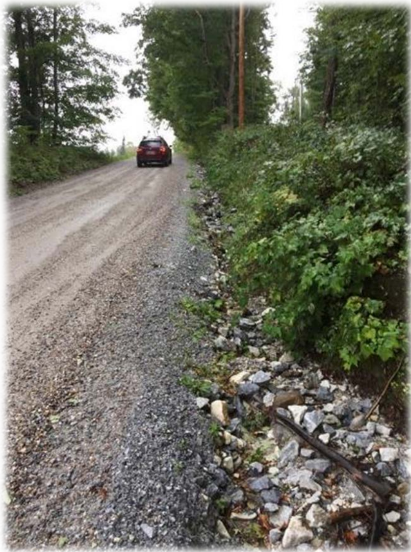
Figure 11: West Hill Road 3. Grader berm needs removing and the ditch is eroding.
