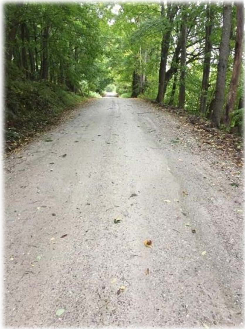
Figure 9: West Hill Road 4. This road segment needs to be re-crowned.
